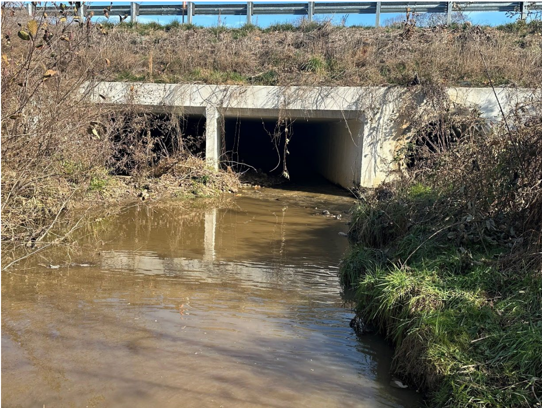
Downstream of Confluence of UT Hyatt Mill Creek with Hyatt Mill Creek entering culver inlet. Division Forces cleared sediment to allow flow through main channel culvert (right barrel).
